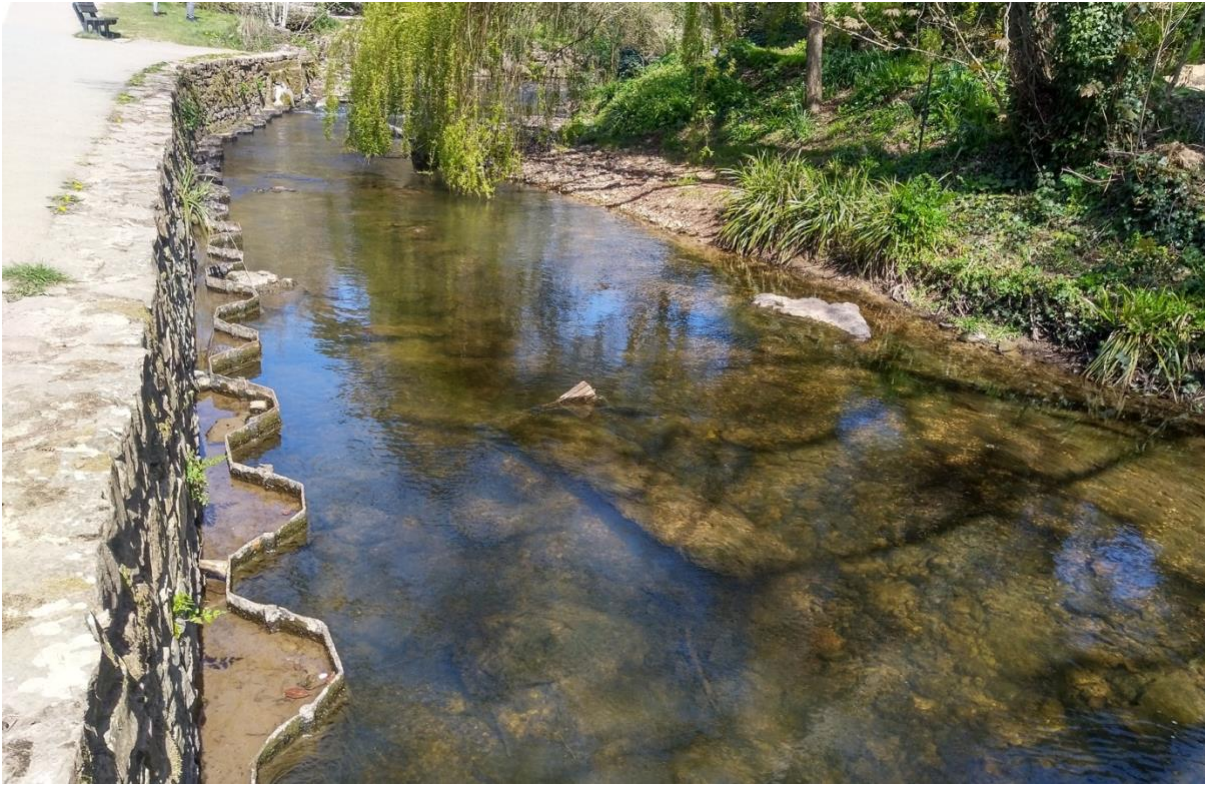
Figure 13 Hard sheet piling revetment prevents the footpath from eroding. Reducing stream energies upstream will allow for a softer, greener bank to be installed. Note the smothered gravels caused by the impoundment of the old weir downstream. SY 12963 88595
