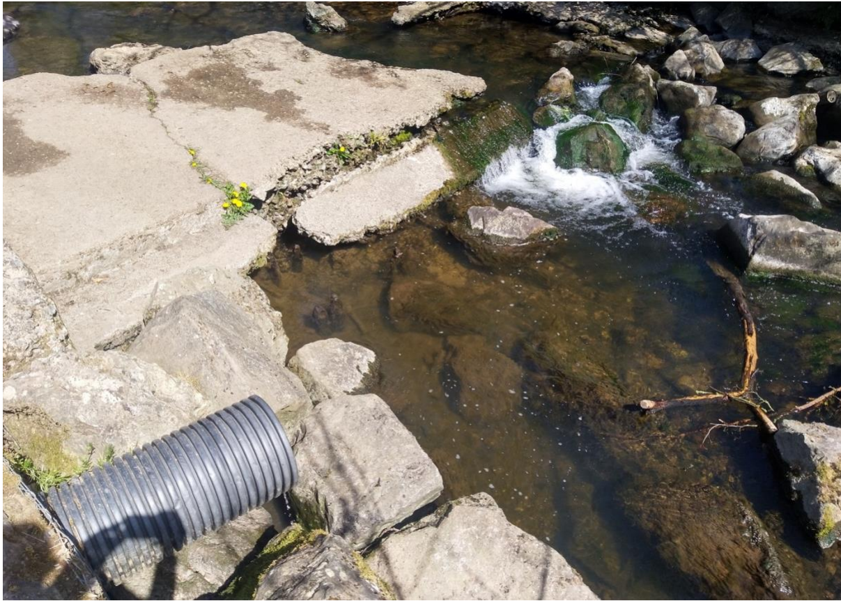
Figure 15 Sewer Storm Overflow Permit No: 201828 no spill duration monitoring available. Algal growth suggesting excessive nutrients in this area. SY 12956 88575
