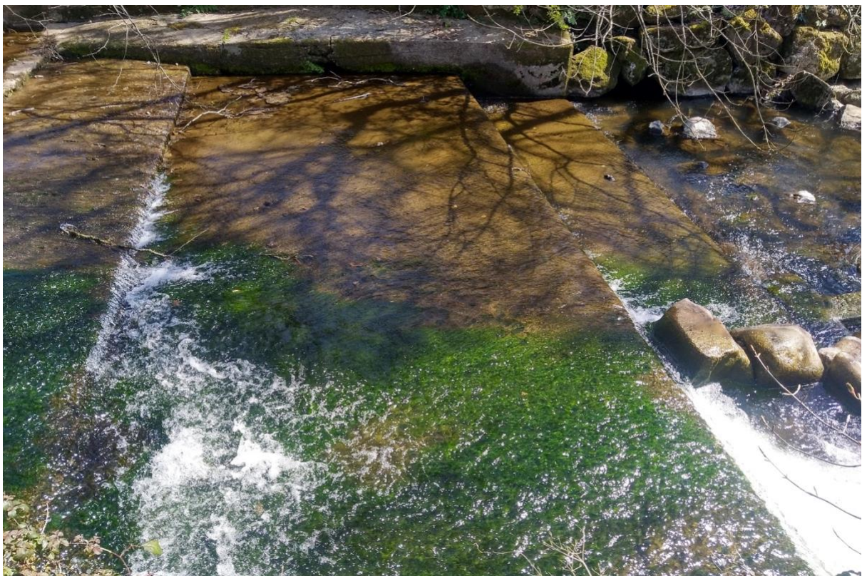
Figure 18 The three shallow steps downstream of the weir in Figure 17. In low to medium flows, there isn't enough water for fish to swim upstream. SY 12969 88498
