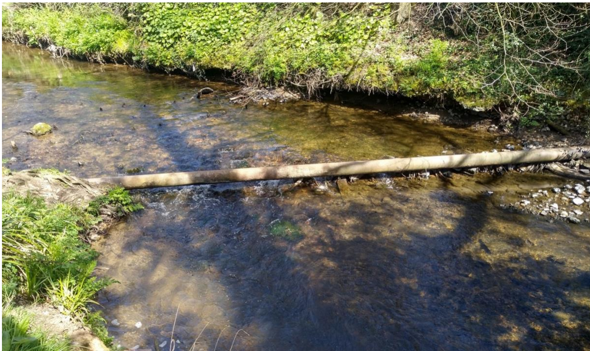
Figure 16 A sewerage pipe crosses the river. With high flow velocities common, this is vulnerable to fracture by passing debris. The asset owner is liable for the environmental damage such a fracture will undoubtedly cause downstream. Liaison with the owner to find a re-routing solution is advised. SY 12977 88539
