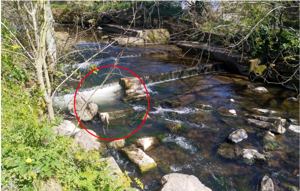
Figure 19 Looking upstream to the weir in Figures 17 & 18. A notional jumping pool has been created to ease the first step (red circle), but overall insufficient to allow good upstream fish passage. SY 12969 88498
