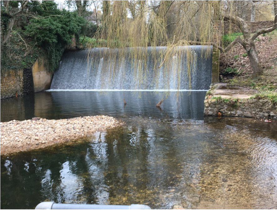
Photo 2 School Weir fish and eel barrier
