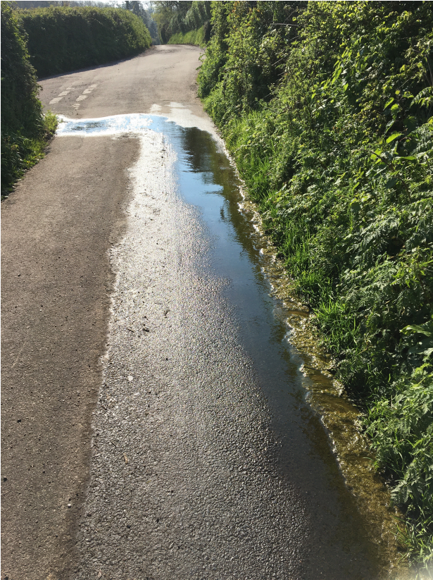
Photo 7 Nutrient rich run off full of algae drains across the Mutersmoor Road and into Bickwell Brook.
